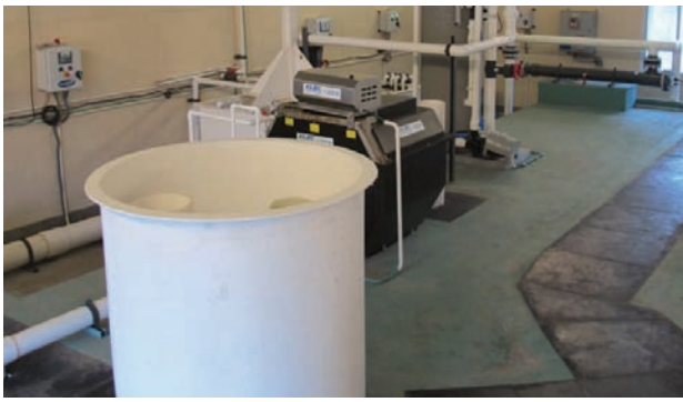
Imported RAS components (Sump, Drum filter & Protein skimmer)
