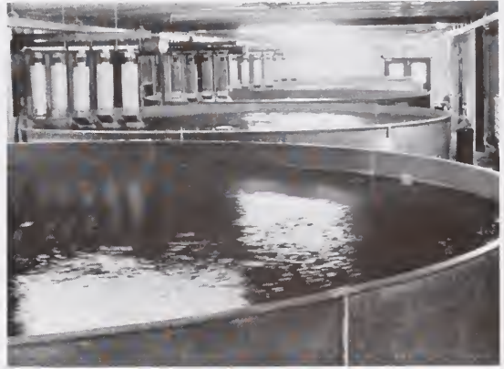
Tank wing of hatchery with degassing columns hanging from the horizontal pipes. Each tank is 20 feet in diameter and has a 12,000-gallon capacity.
