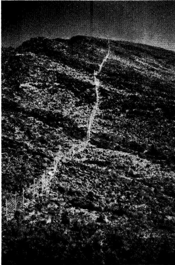
Figure 19. Newly constructed fence in upper Kahikinui district, south boundary of Haleakala National Park, to prevent ingress of feral goats and pigs. Photo by Peter Sanchez, National Park Service, January 1985.
