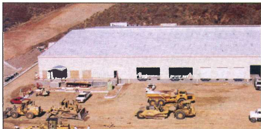
Construction will soon be completed at the new state-of-the-art spring water bottling facility on the San Manuel Band of Mission Indians Highland reservation.
