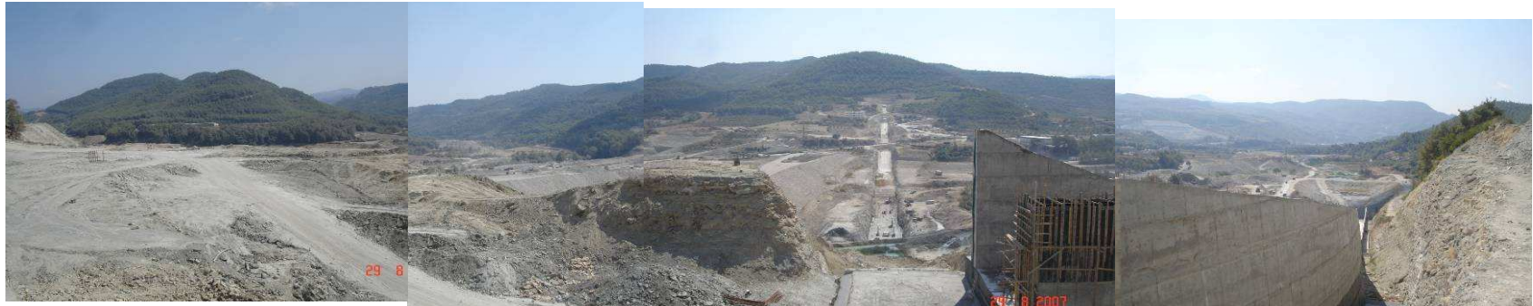
Photo 51: The infrastructure projects destroyed wide areas from the forest as the case of Paradon Dam project on Al-Shamali River
