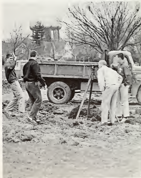
The Sigma Chis carefully watched the early stages of the construction of their new addition.
