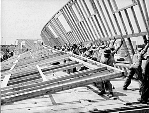
Figure 1 The balloon frame being erected in the 1940s. Built with 2x4 inch dimension lumber, cut and butt-jointed and fastened with nails. The structure is redundant and each joint is reasonably solid such that the entire system has a statistical probability of sufficient bearing capacity.
