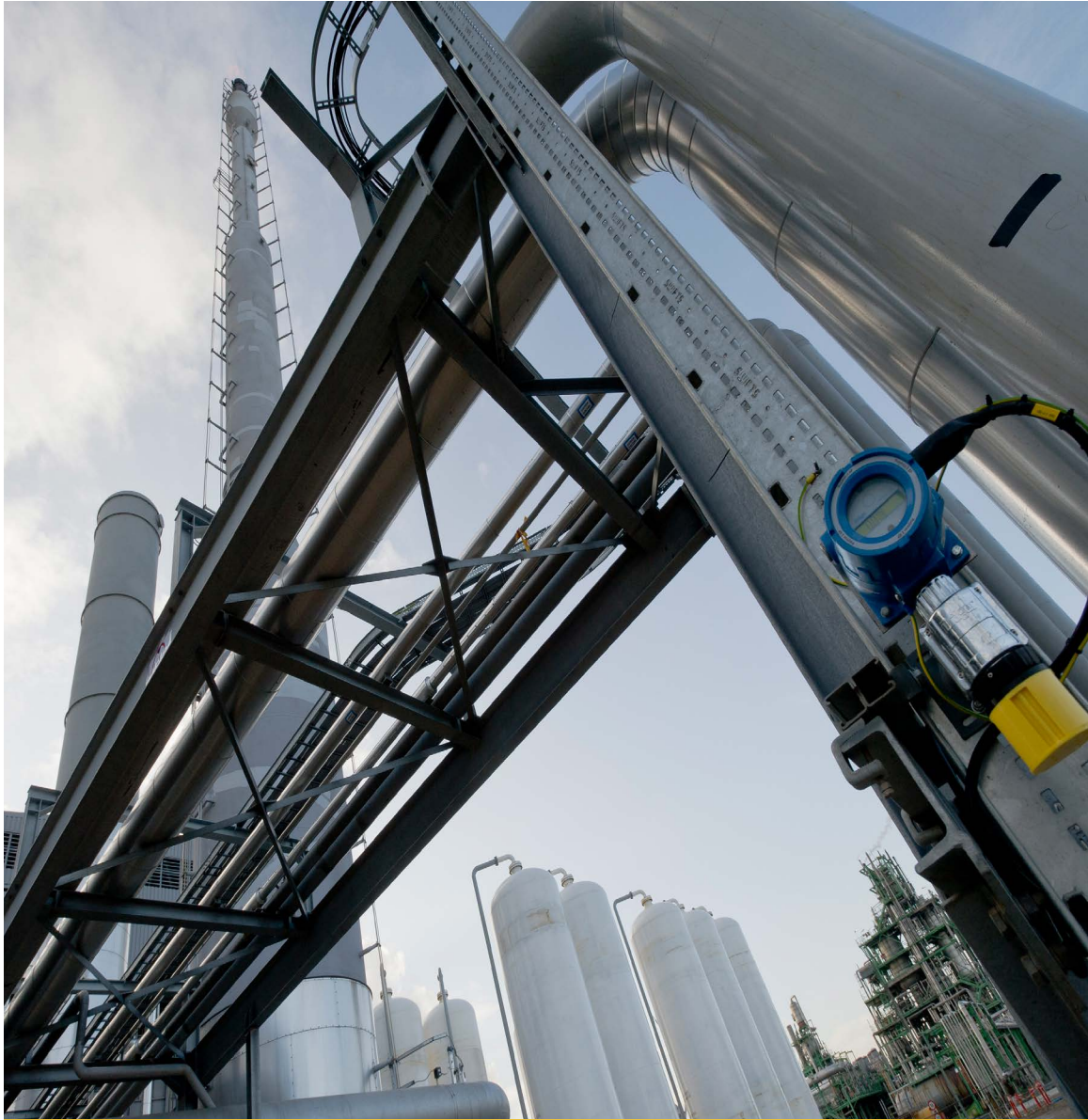
ExxonMobil and Air Products partnered to construct this hydrogen production plant in Rotterdam, the Netherlands.
