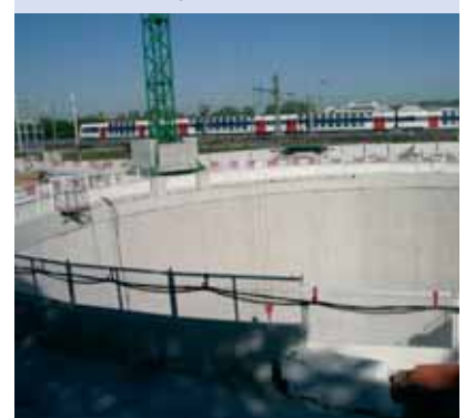
Emergency shaft and ventilation unit near the RD10 (Viroflay)
