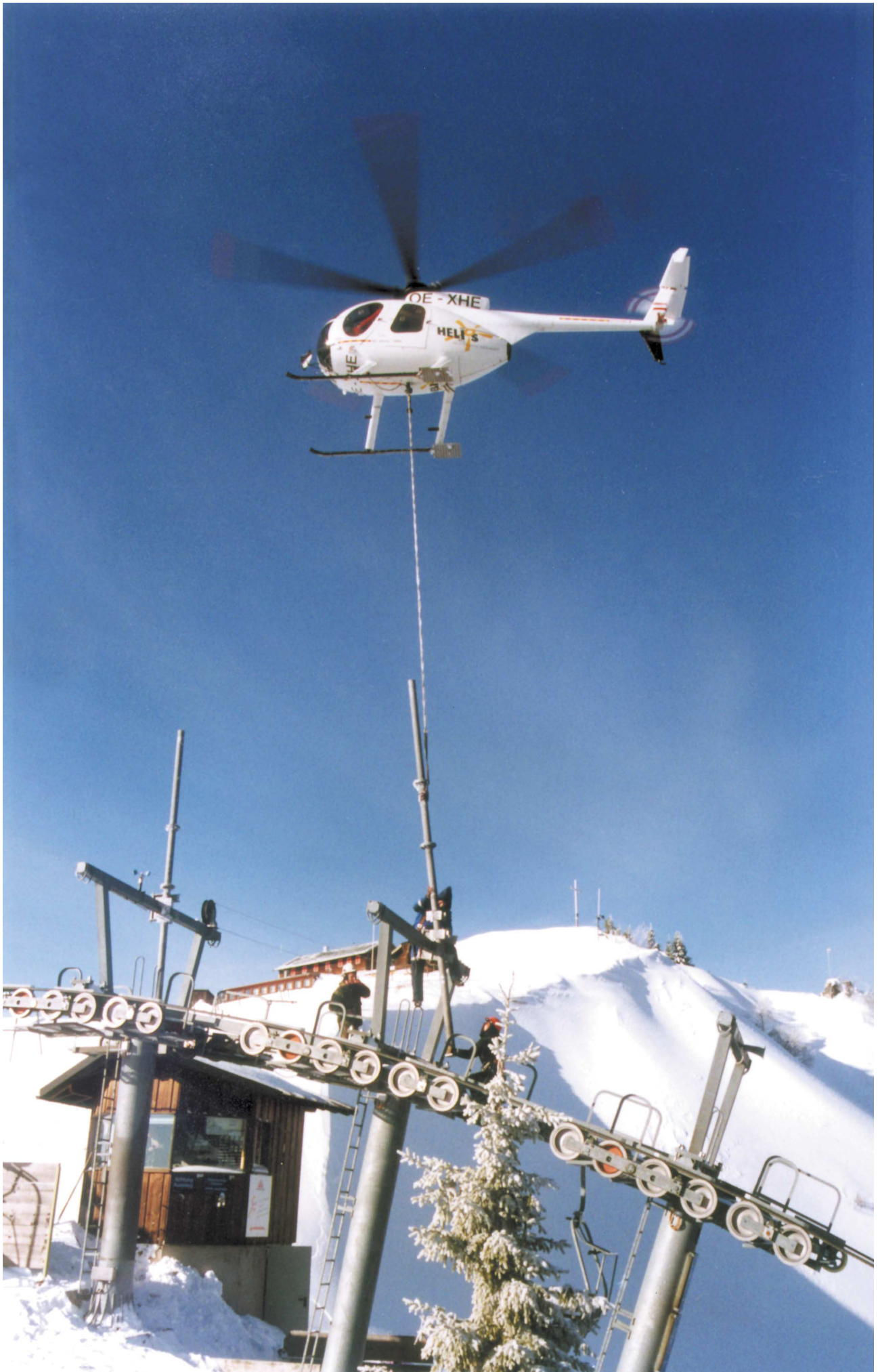
Installation of a new antenna pole with a helicopter at the skiing area "Brauneck" Bavaria/Germany.
