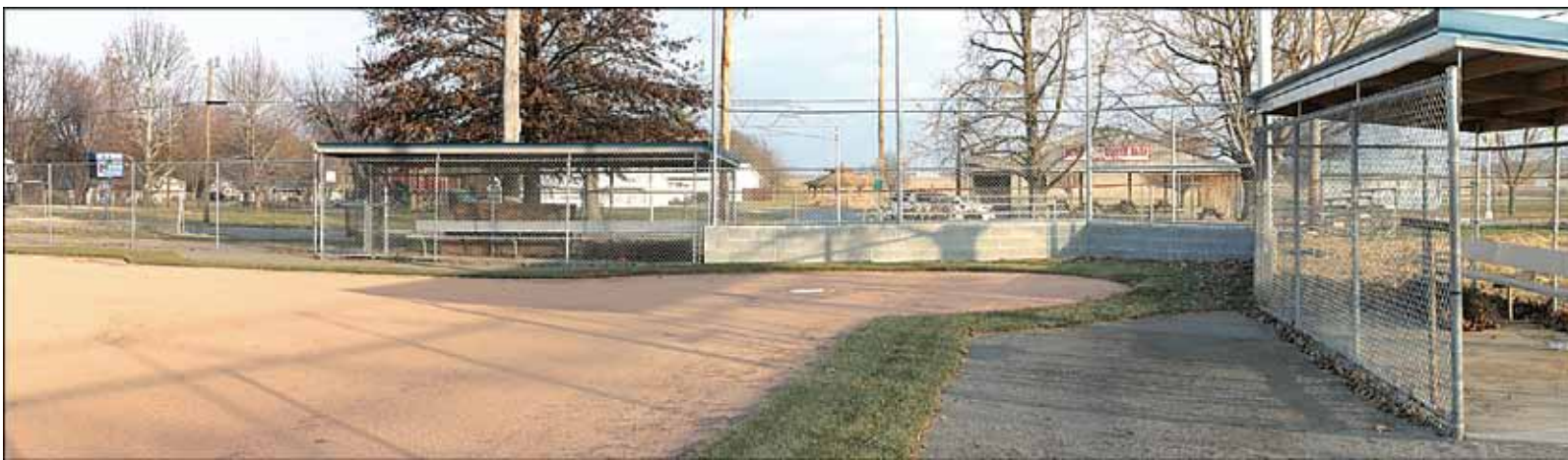
This photo shows the expanded dugouts, a portion of the new infield surface and the concrete block and screen backstop at main ball field in Ava. The renovations were made possible with the help of a $10,000 grant from the Elizabeth Smysor Trust Fund and many donations of materials and volunteer time.
