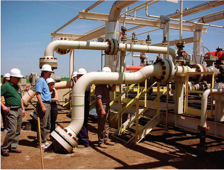
FIGURE 6 A portion of the pipeline delivering CO 2 to the Weyburn oil field in Saskatchewan, Canada. PHOTO COURTESY OF IEA GREENHOUSE GAS PROGRAMME
