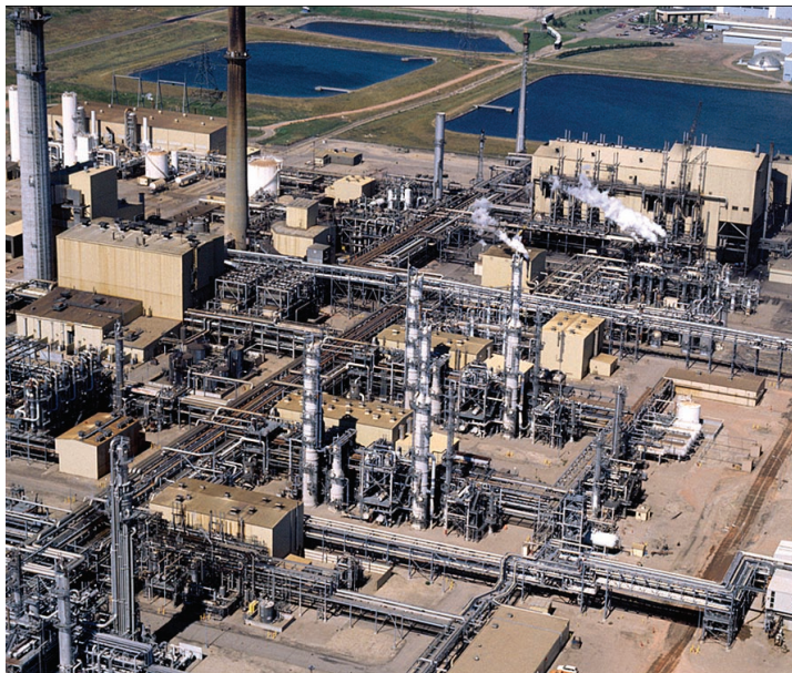
FIGURE 4 A precombustion CO 2 capture system used to produce synthetic natural gas (syngas) from coal at the Dakota Gasification Plant in North Dakota. About 3 Mt/y captured CO 2 is currently transported by pipeline to the Weyburn and Midale oil fields in Saskatchewan, Canada, where it is used for enhanced oil recovery and sequestered in depleted oil reservoirs. PHOTO COURTESY OF U.S. DEPARTMENT OF ENERGY
