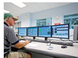
Central Room Monitoring
