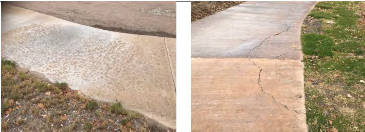
Figure 9. Example of erosion (left) and surface cracking (right) on paved trails in LPSP.
