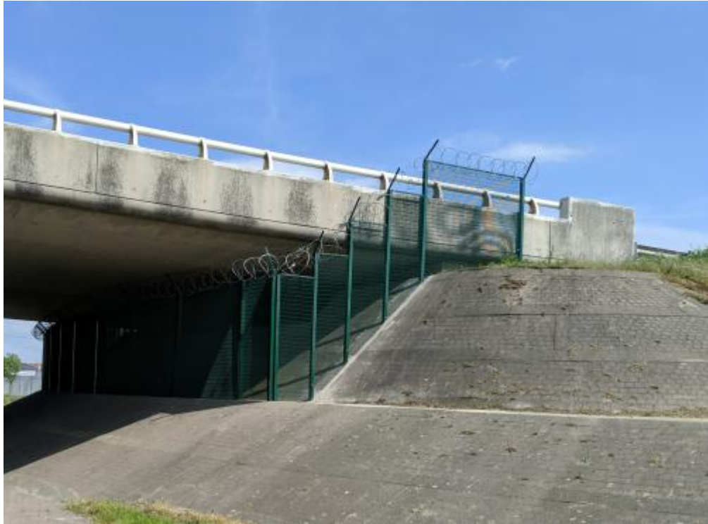
FIGURE 23: Fencing underneath N216 motorway bridge close to Zone du Marcel-Doret . Installed February, 2019 (Boussemart, 2019a). Author's photograph taken April 2019.
