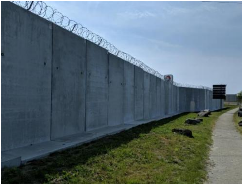
FIGURE 2: Wall surrounding Total Transmarck where migrants stow-away on UK bound lorries. Author's photograph September 2019.
