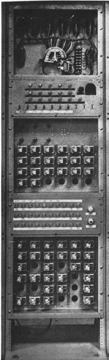
CONTROL-SYSTEM panel at left distributes commands to banks of relays in three panels at right, one for
