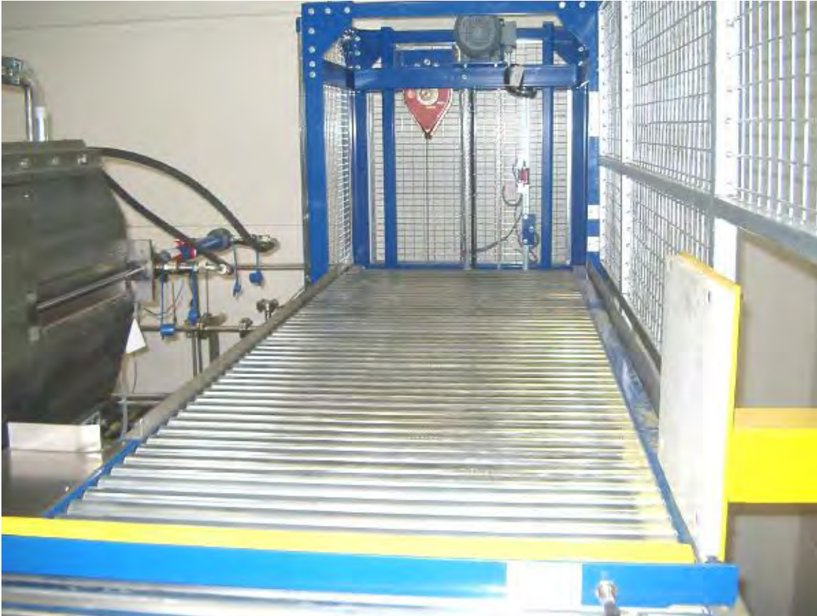
Figure 2-5: Exit of Feed Elevator to Apron of First Loading Chamber
