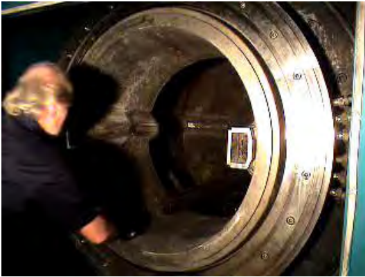
Figure 3-7: Opening of SDC Chamber in Inspection Position
