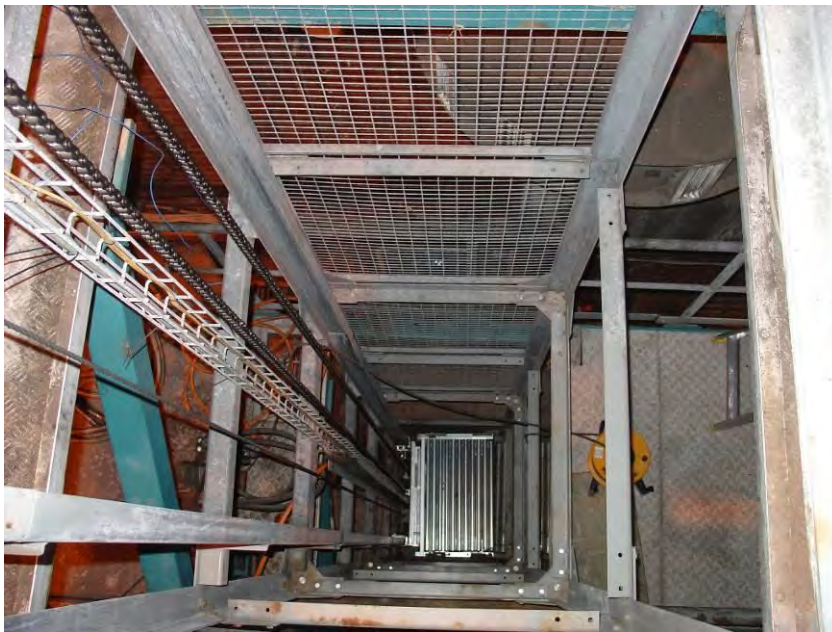
Figure 4-17: Feed Elevator Looking Down from Top Level
