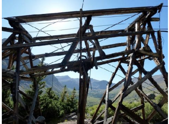
Magnolia tram tower, looking west toward the headwaters of the Middle Fork.
