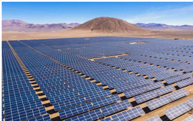
Huge photovoltaic plant in the Atacama Desert, Chile
