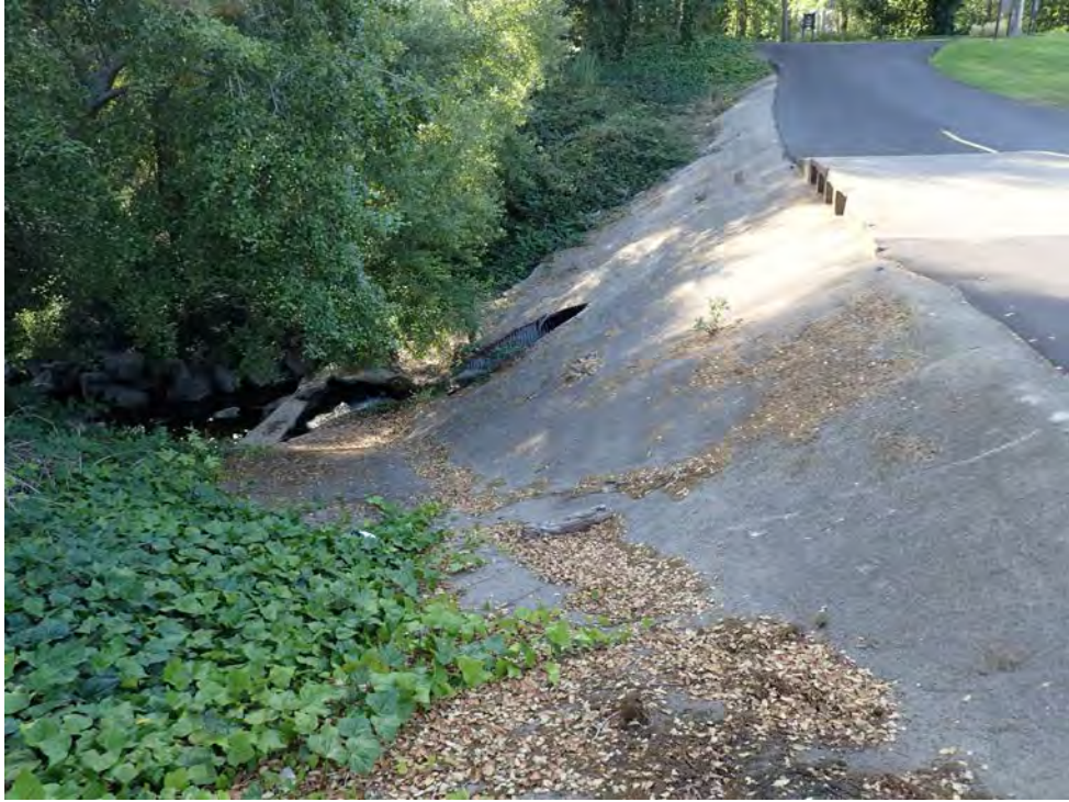
View from the top of the summer impoundment dam looking towards the downstream culvert.
