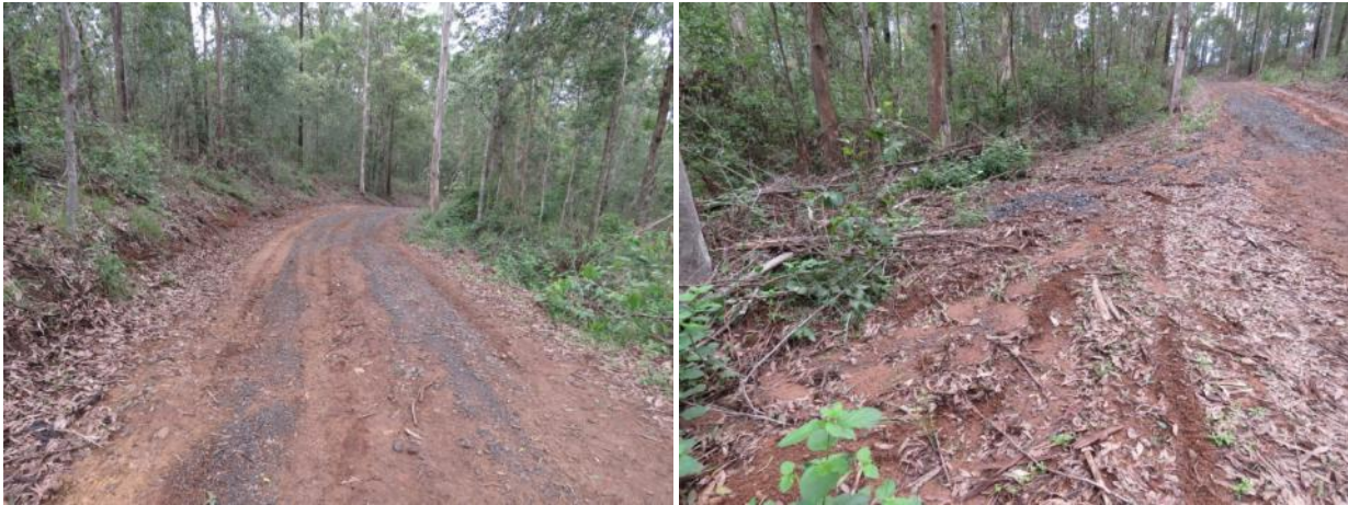
Mangrove Creek Road in adjacent compartments, showing gravelling, upgrading and erosion.
