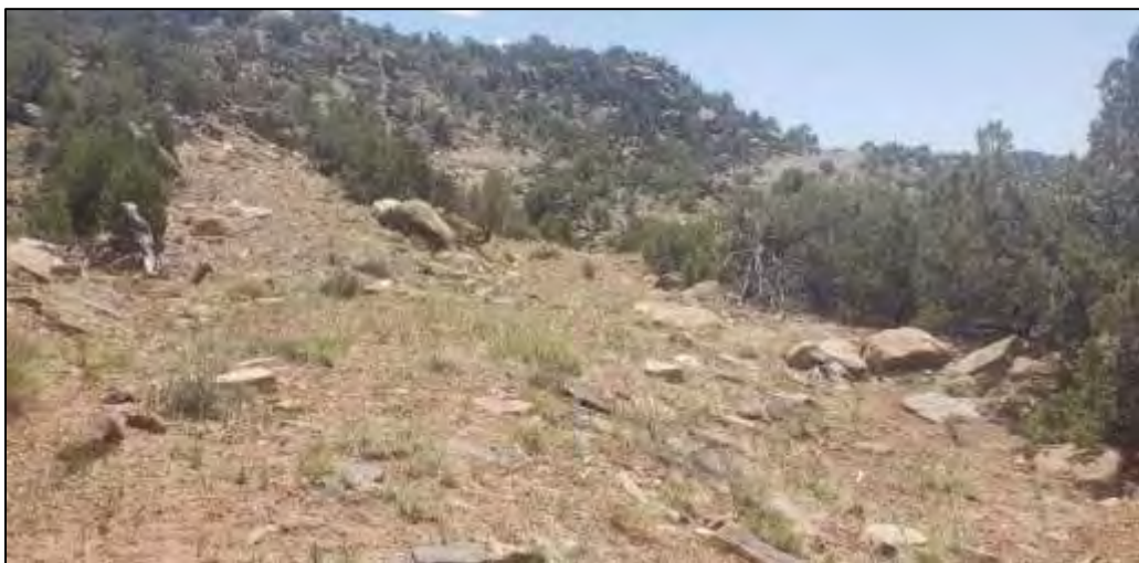
Figure 16. This photograph was taken at SDH5 and is looking south across the reclaimed portion of the road.
