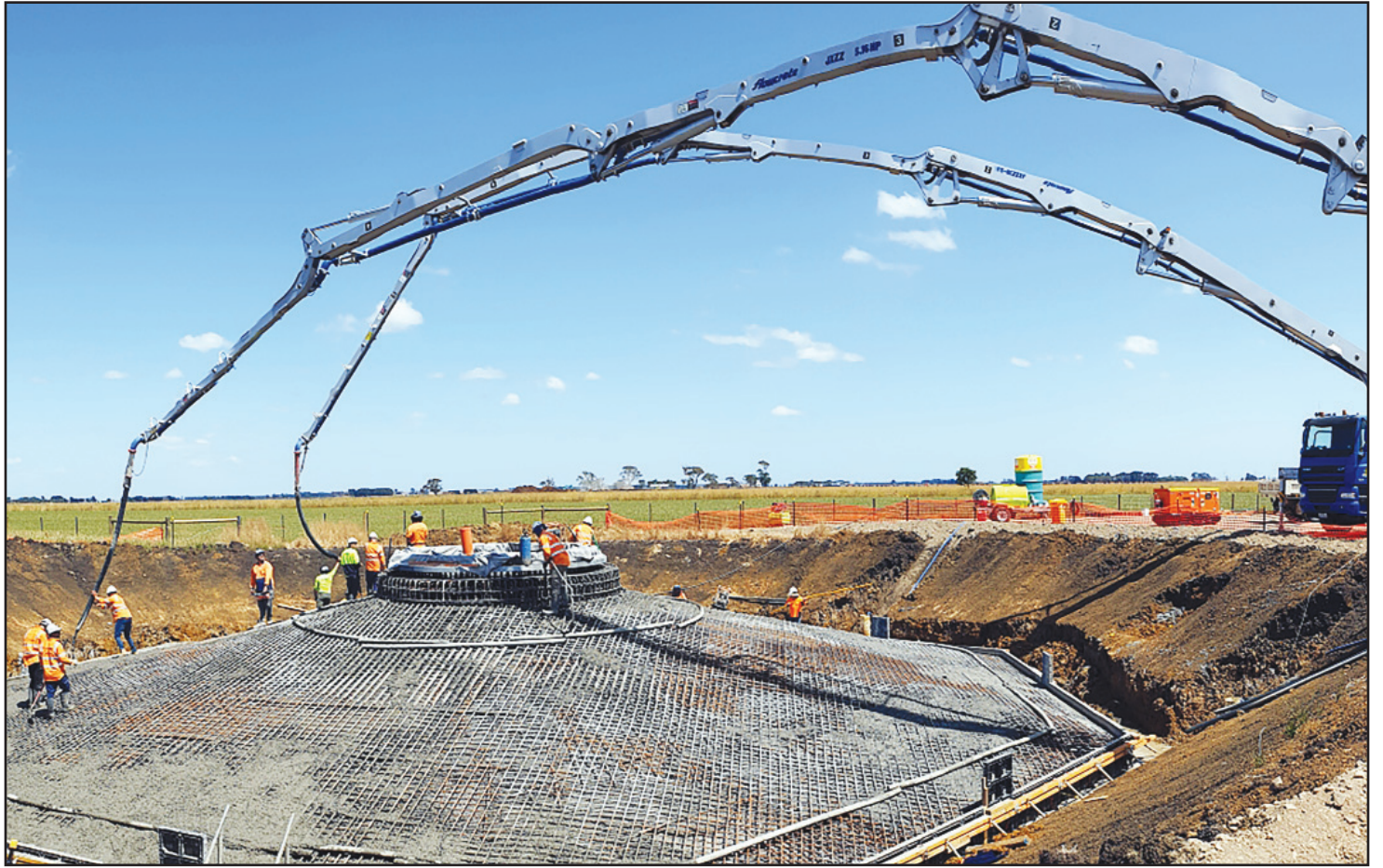
Nearing completion: The Mortlake South Wind Farm project team saw another milestone achieved, with the last of the 35 turbine foundations poured last week. 2020E
