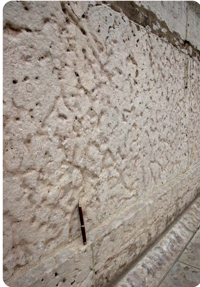
Feeding burrows produced by an unknown type of animal, preserved in an exterior wall of the Statehouse. In places (such as at top right of this photo), Statehouse caretakers have filled exposed burrows with grout to reinforce the facing.
