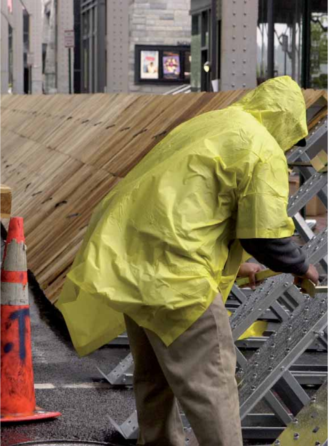
Workers construct a flood wall to protect buildings in the United States. Source: FEMA/Liz Roll.
