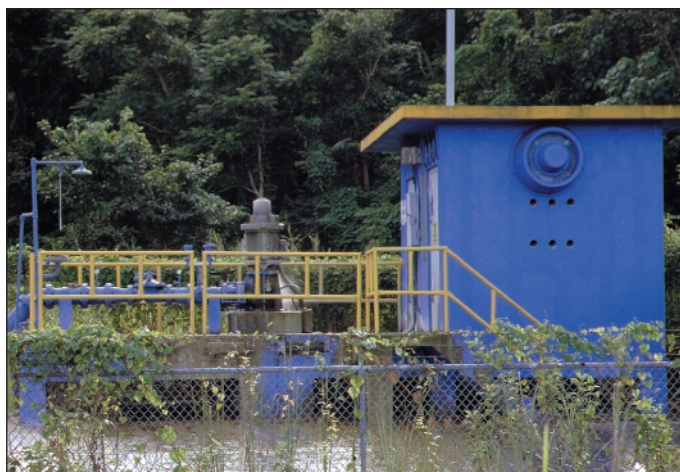
Photo 51. The Puerto Rico Water Company's ground water pumps in Dorado, Puerto Rico. Photo by L. Miranda Castro.
