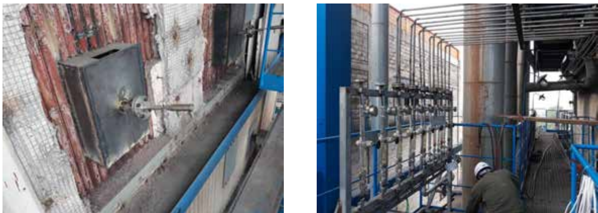
Figure 4.10 SNCR system Installation
