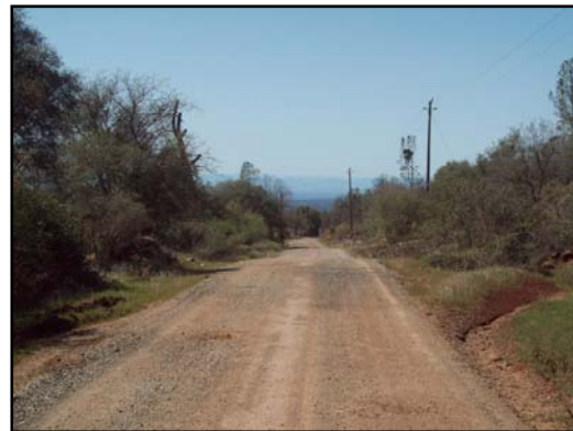
Battle Creek Bottom Road, eastern end: Note dense brush to the road edge.
