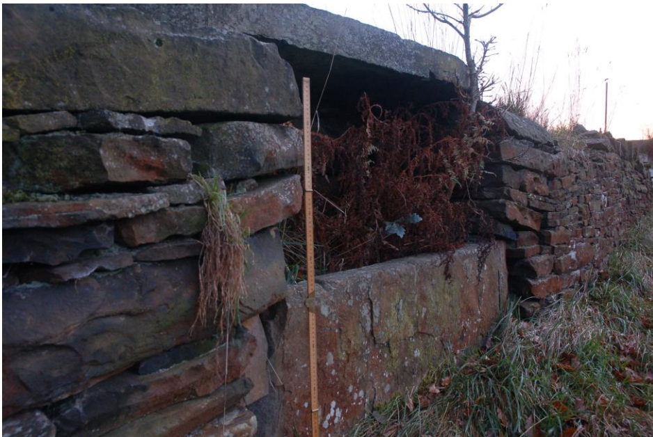
Figure 2 Tan Well, Hebden Bridge. This trough is recessed into the wall and surmounted by a segmented arch, as are a number of others in Upper Calderdale. There is a bung-hole in the front of the trough which, if stoppered, would raise the level of the water within.
