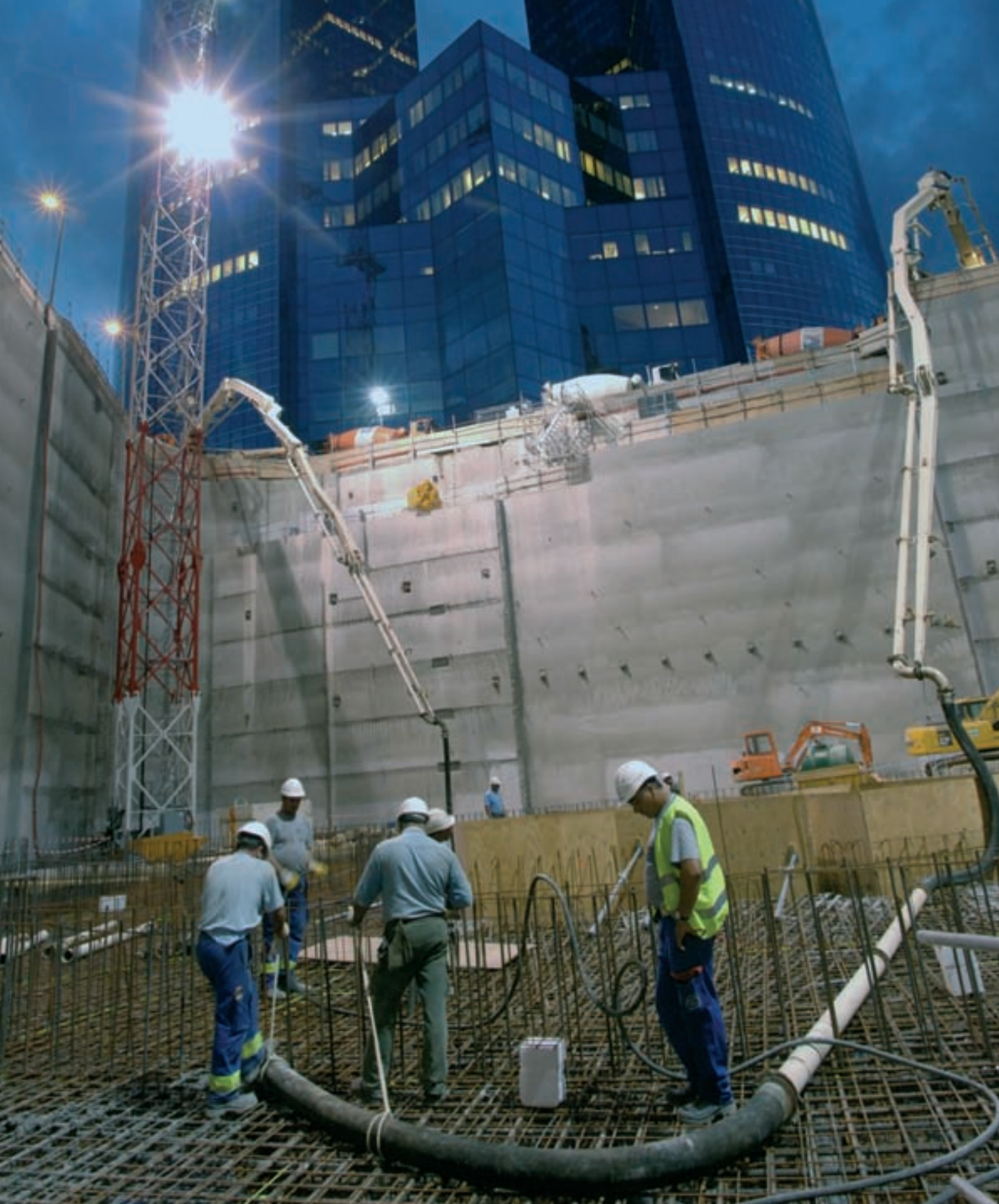
Above. The Granite tower under construction for the Société Générale in the La Défense business district will be the first High Environment Quality® certified high-rise building. For VINCI, this worksite is also serving as a laboratory - researchers are carrying out safety-related behavioural studies there under Vigisite auspices.
