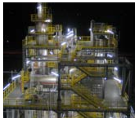
Hostalen ACP technology plant at Basell Orlen Polyolefins joint venture in Poland
