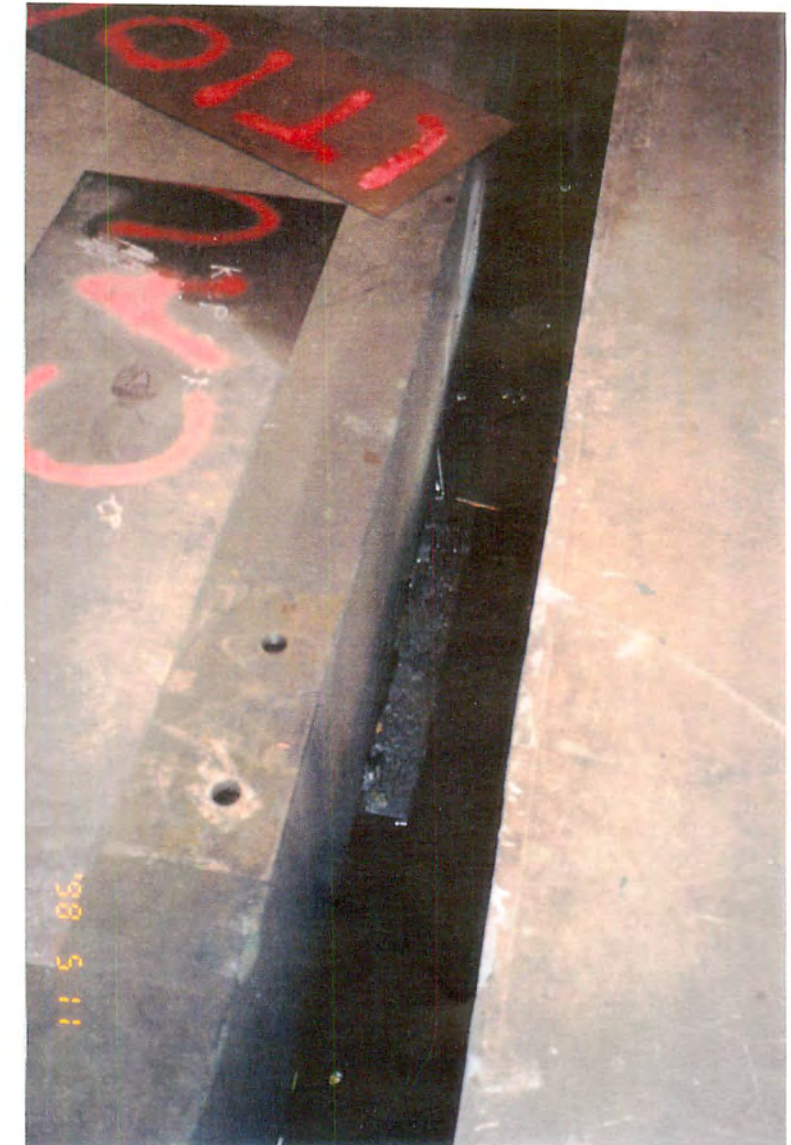
FIGURE 13: 1 x 15 FT PIT IN NORTH MIDDLE BAY, PROBABLY PART OF A REMOVED HOIST ASSEMBLY. PIT CONTAINS APPROXIMATELY 30-50 GALLONS OF HYDRAULIC OIL.
