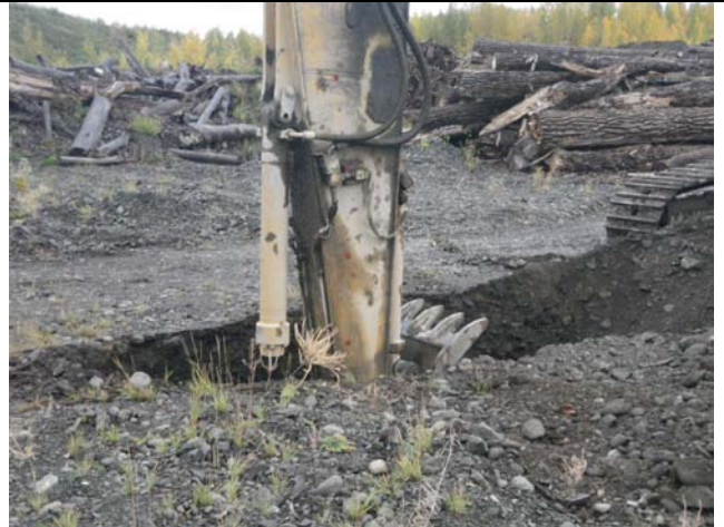
Photo 2. Test pit depth estimated based on scale on excavator arm (red dots)
