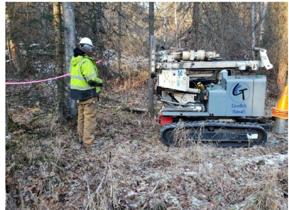
Monitoring well installation as part of EPA area-wide assessment grant to the Municipality of Anchorage
