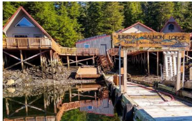
DBAC services conducted at Jumping Salmon Lodge included assessment, HBM inventory, and a drum and tank inventory, Chenega
