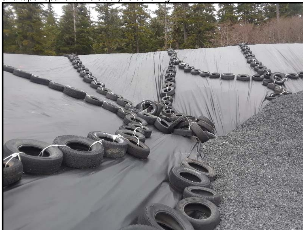
Photo 10: Looking north at the treated stockpile prior to investigation. Note the tires piled up near the toe of the stockpile slope which resulted when snow load on the stockpile shifted the securing "tire chains" during the winter/spring of 2018.
