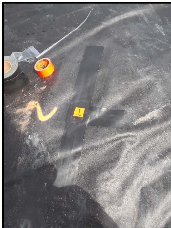
Photo 9: Looking down at pore water sampling point W1 after cutting and capping the PVC casing and tape repairs to the stockpile covering.
