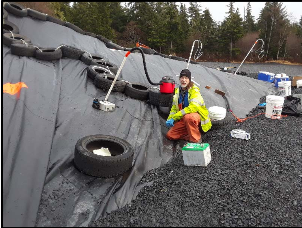
Photo 3: Looking east at sampling point W3 at the Byford Junkyard Site. Note vacuum suction being applied to sample point in attempt to draw additional pore water for sample collection.
