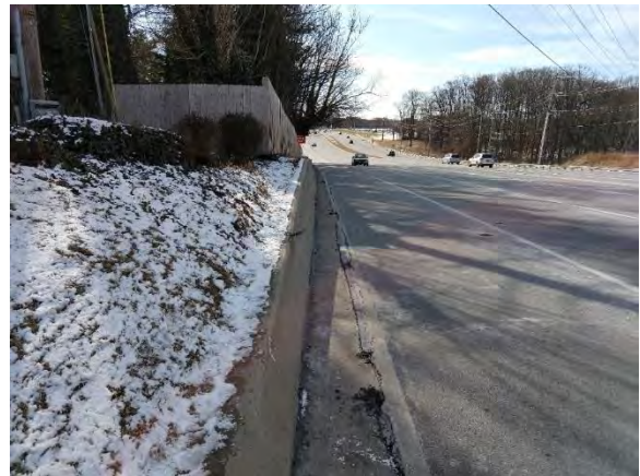
Missing sidewalk along NB US 202
