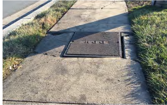
Horizontal gap at utility cover
