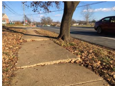
Elevation difference due to tree roots
