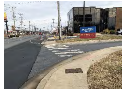
Missing signal heads at Mt. Lebanon intersection
