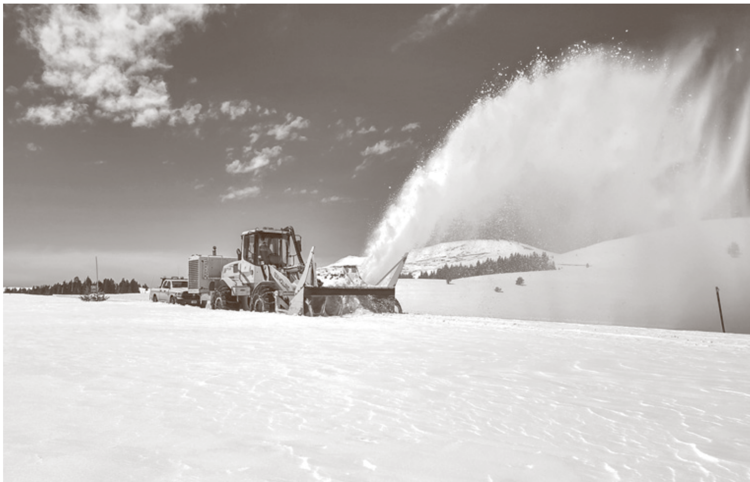
Lovell heavy equipment operator Rick Gurney operates a snow blower on top of the Bighorn Mountains during the annual opening work of U.S. Highway 14A east of Lovell in early May. Photo courtesy WYDOT
