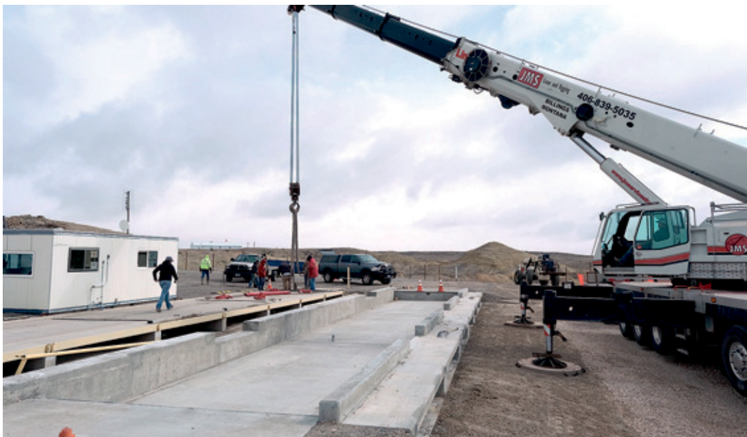
A heavy crane was brought into the county landfill site southeast of Powell to lift existing scales off the old foundation and place them on a new one. The landfill is located on Road 5. Tribune photo by Eric Gill
