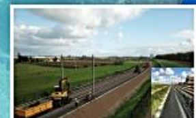
Construction of an inspection pathway over 46 km alongside railway track Hoekse Lijn.
