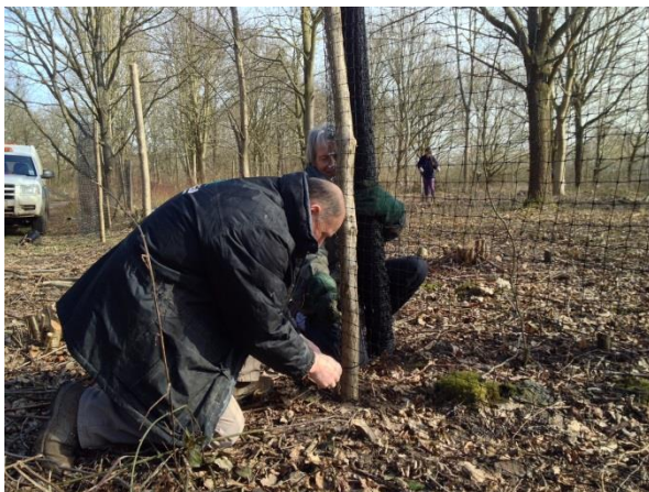
Horton Country Park LNR volunteers erecting deer fencing at Sherwood Grove winter 2015
