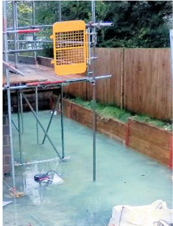
Figure 32: Example of a development in the Littleton district. The building had trenched into the hillside in an area normally dry. The excavation breached the water table in the chalk aquifer during a period of high groundwater.
