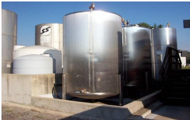
Secondary containment at a bulk pesticide facility.
