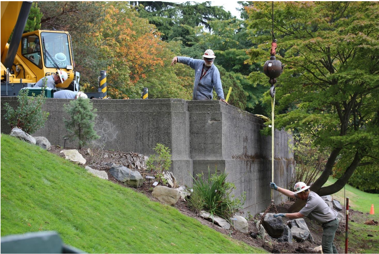
Figure 41 Lock and Dam mechanic Steven G. Hansen signals crane while gardener Stephen J. Munro places boulder October 2017. Michelle K. McMorran
