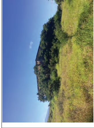
Photograph 2: Exterior view of concrete structure located on the north portion of the Subject Property.
