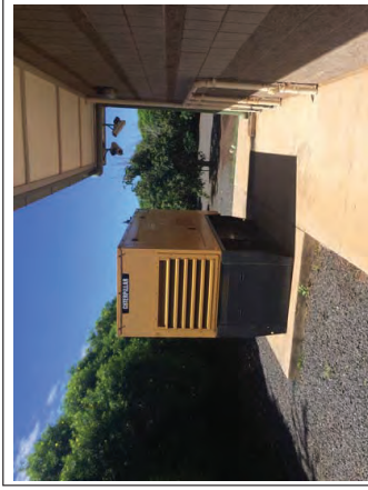
Photograph 8: View of generator located on the east portion of the telecommunication station.
