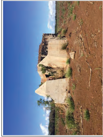
Photograph 17: View of one of the concrete bunkers located on the north portion of Parcel 34 (Field 916).
