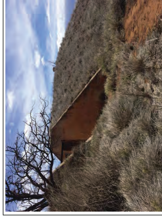
Photograph 14: Exterior view of one of the bunkers located on the north portion of Parcel 34 (Field 916).
