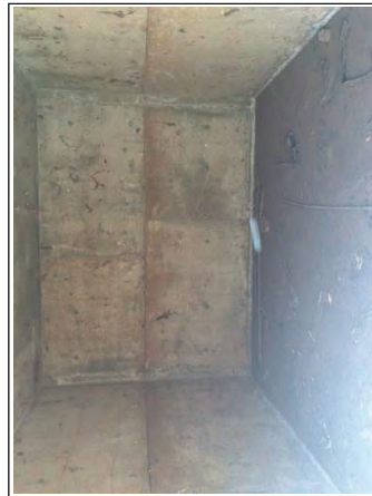
Photograph 18: Interior view of one of the concrete bunkers located on Parcel 34 (Field 916).
