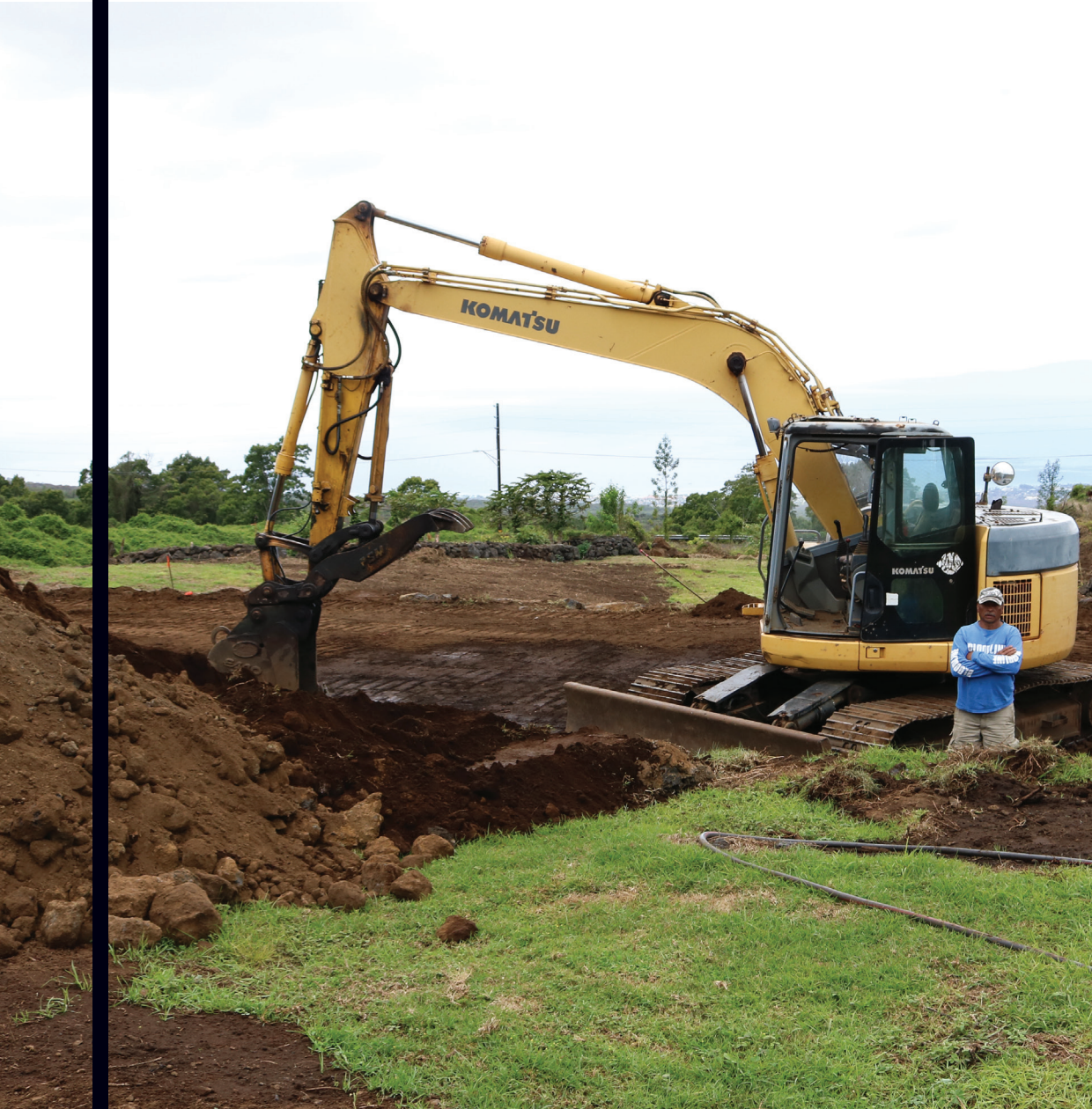
▶ Waiohuli lessee taking a break from operating an excavator as he prepares his homestead lot for a new house.
