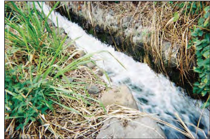
Figure 14: Site 50-50-04-5729 Ditch, Showing Rock and Mortar Construction of Side Walls. View to Northwest.
