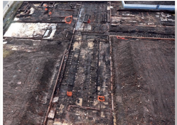
High-level view looking south, showing the remains of the track bed for the travelling crane
