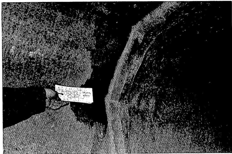
Photograph 10 Showing the same culvert roof after three years exposure to sulphuric acid attack.
