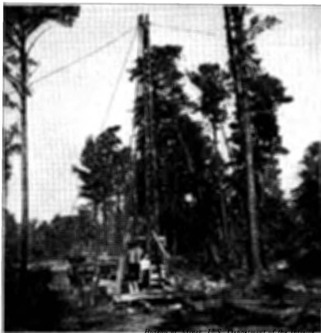
Bureau of Mines, U.S. Department of the Interior Figure 5. Rig used to drill no. 1 churn-drill hole. Note 18-inch bit in foreground and bailer standing upright at left of rig
