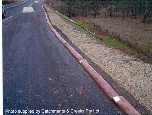
Photo 2 – Sandbag flow diversion berm used to minimise surface flow over a recently seeded embankment
