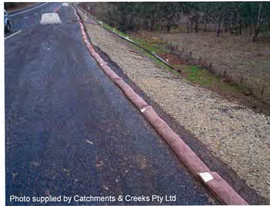
Photo 4 – Sandbag flow diversion berm used to minimise surface flow over a recently seeded embankment
