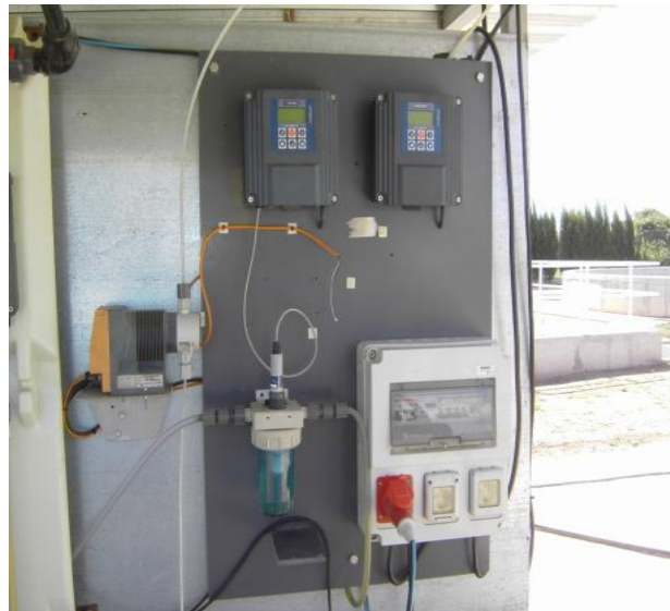
Figure 5. View of the peracetic acid system.
