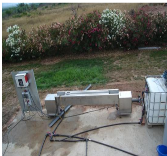
Figure 6. View of the peracetic acid system.
